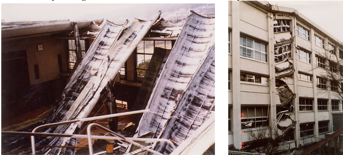
Source: Architectural Institute of Japan (AIJ), Damage Investigation Report on Reinforced Concrete Buildings due to the 1995 Hyogoken-Nambu Earthquake -Part II School Buildings- , 1997.
